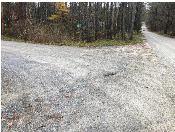
Photo 1: Runoff is eroding the roadway and bypassing an existing turnout on Trumbull Hill Road near the Oak Hill Road intersection.
